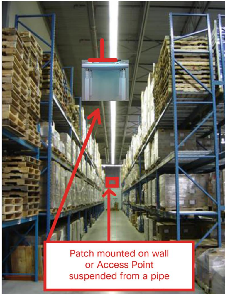
Figure 33. AP Placement in warehouse environment
